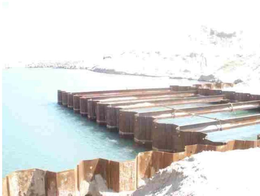
Temporary Sheet Piles were Erected in Sea Water Intake North Side for Commissioning Purpose
